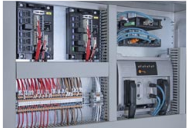
ifm's ecomatController for mobile applications (bottom right) is mounted in the control cabinet outside the vehicle.
