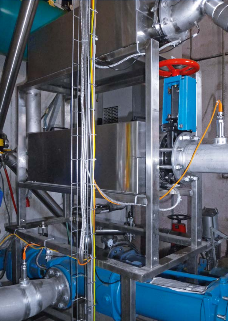
In the ultrasonic disintegration plant, biomass is processed for maximum energy yield.
